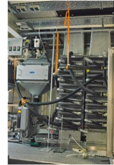
Blower, filter, Heat exchanger
